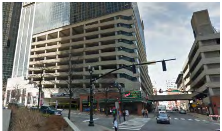
Inappropriate upper level facade treatment
