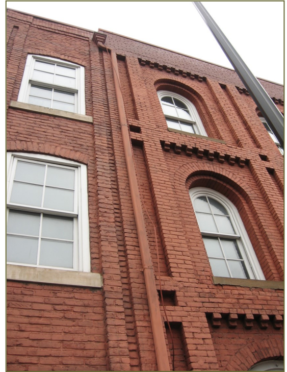
Downspouts on front or side façades should be painted to blend with the paint or masonry color.
