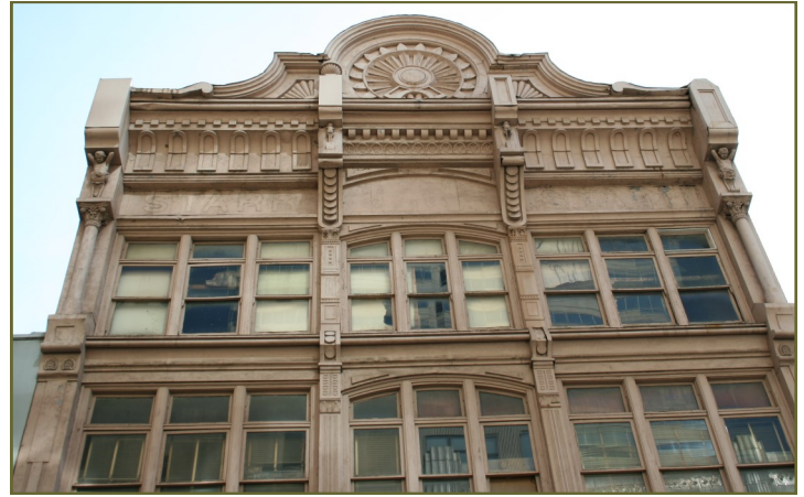
The cornice at 250 Fourth Avenue North is historic; it should be retained and remain visible.
