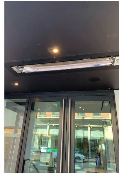
EXISTING LIGHTING FIXTURE
