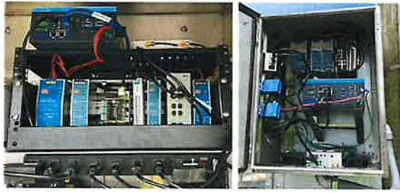
Figure 6. Two styles of pre-fabricated lidar equipment installations developed during Stage I. Left: a drop-in rack mount with lidar equipment, for traffic cabinets with sufficient space. Right: an accessory cabinet affixed onto existing signal cabinets.
