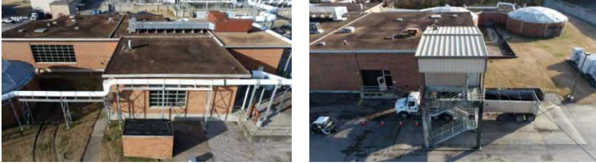
Figure 14-8. Exterior Filter Building Photos Showing Foul Air Ducts and Sludge Load-Out Area.
