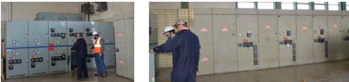
Figure 11-2. MV Main Switchgear (left), MV Blowers MCC (right)
