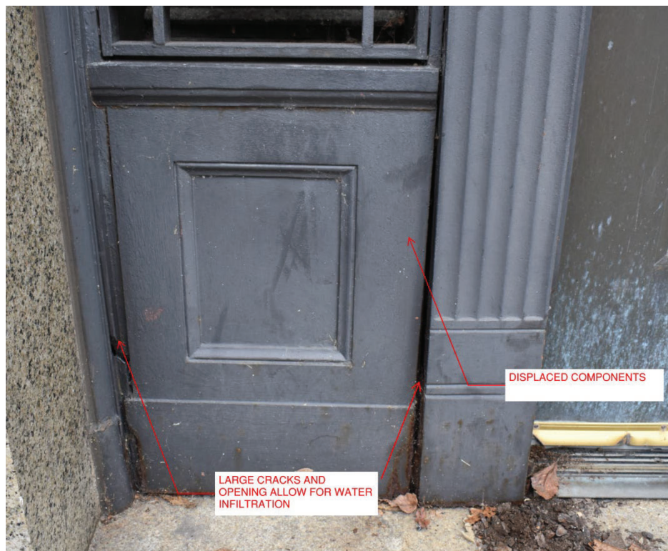
Detail images of severe corrosion and deterioration on cast iron surround elements. Images by TTG.
