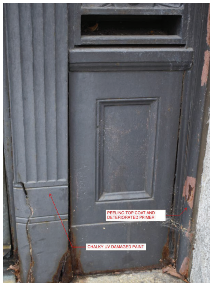
Detail image of paint and sealant coatings that are beyond their service life. Image by TTG.
