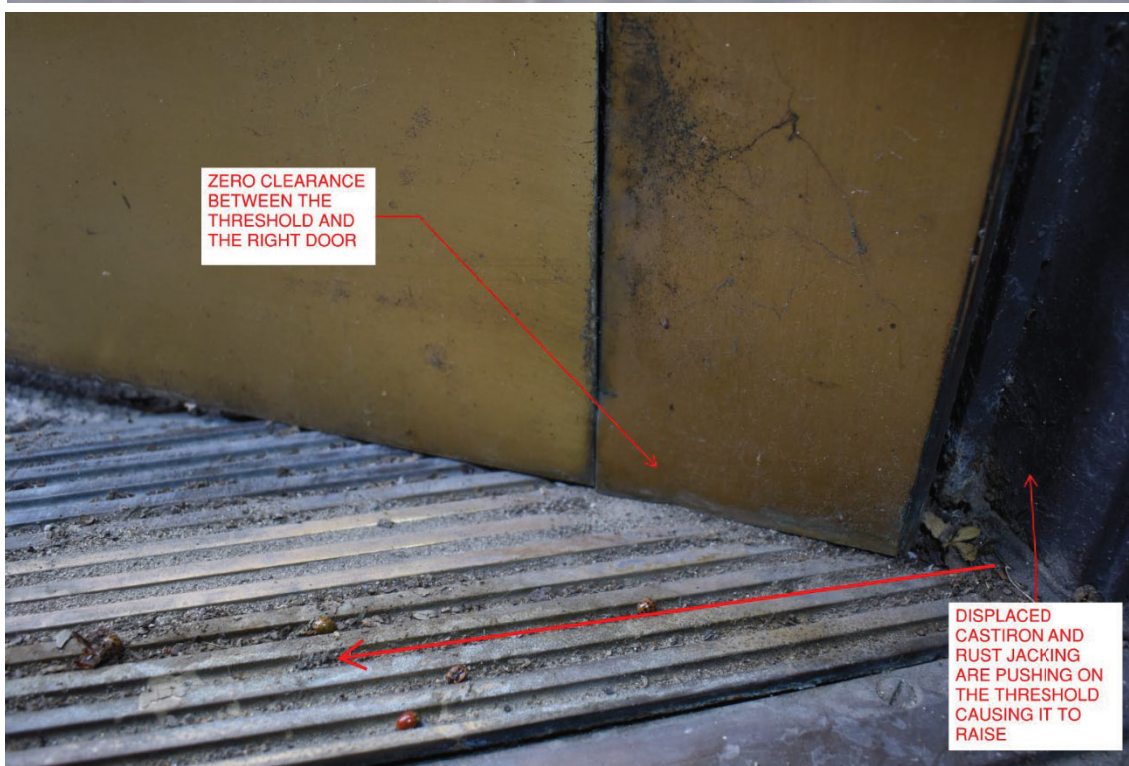
Detail images of deleterious conditions observed on thresholds during the assessment. Images by TTG.
