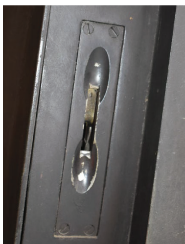
Detail image of the missing bolt lever observed during the assessment. Image by TTG.
