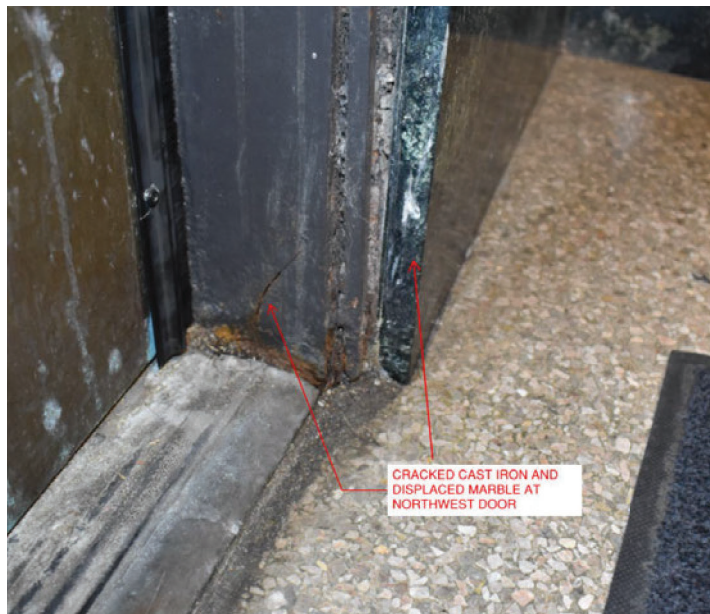
Detail image of cracked and displaced cast iron components. Image by TTG.
