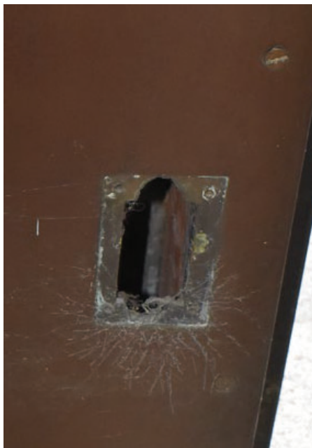
Detail image of a missing receive plate observed during the assessment. Image by TTG.
