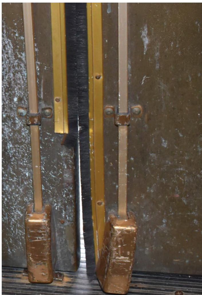
Detail image of deformed weather-stripping on north façade doors. Image by TTG.
