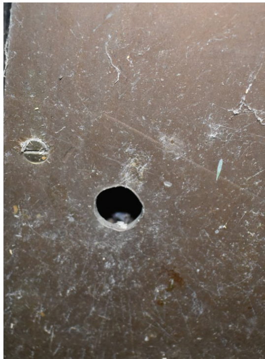
Detail image of one of the holes observed in the cladding during the assessment. Image by TTG.
