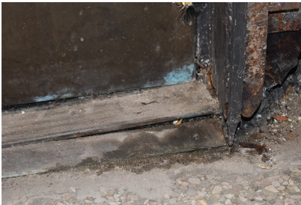
Detail image of deteriorated threshold on the northeast door. Image by TTG.
