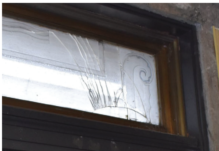
Detail image of crack transom glass. Image by TTG.
