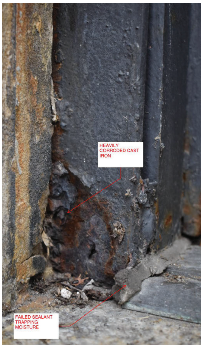
Detail image of heavily corroded cast iron on a door surround found on the west façade. Image by TTG.
