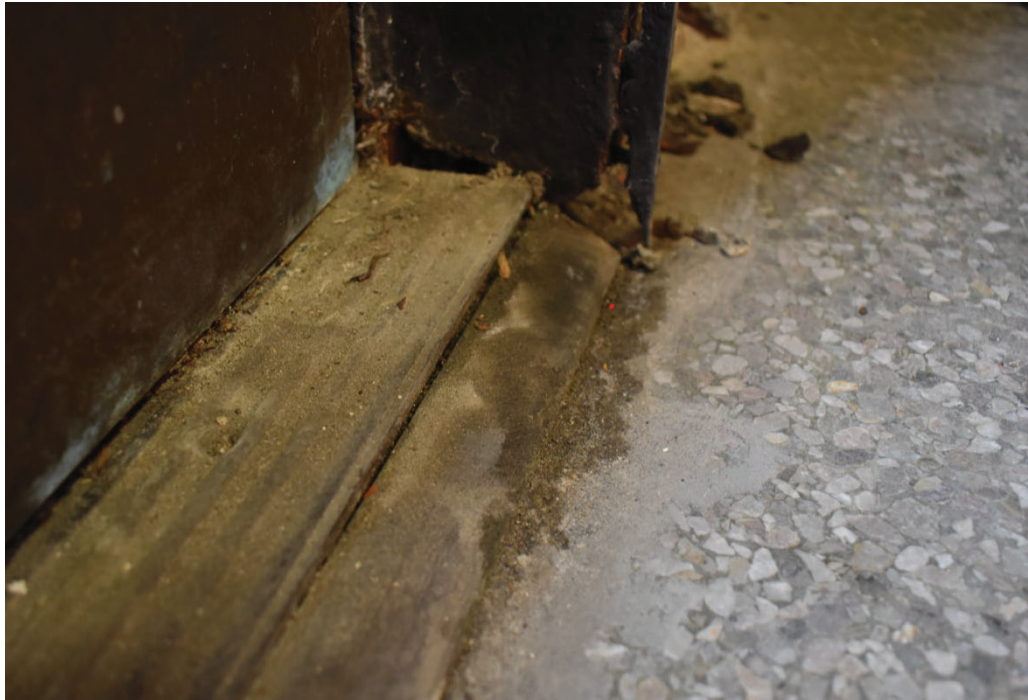
Detail image of deteriorated cast iron members. Image by TTG.
