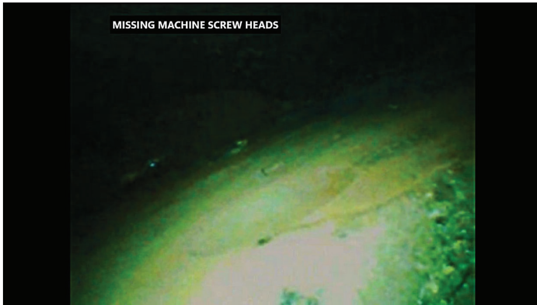
Borescope image that illustrates sheered machine screws. Image by TTG.
