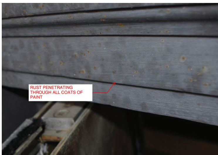
Detail image of paint and sealant coatings that are beyond their service life. Image by TTG.
