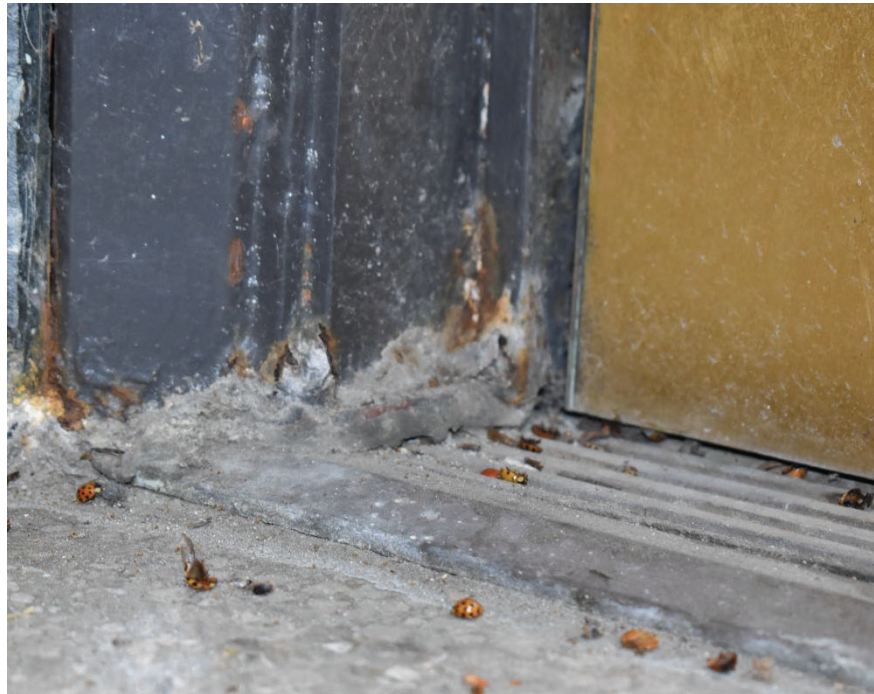
Details images of corrosion displacement and movement on cast iron components. Images by TTG.
