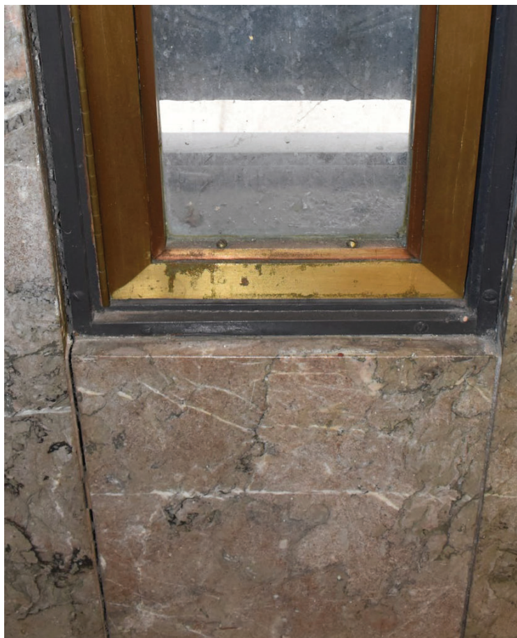
Detail image of water intrusion on a sidelight examined during the assessment. Image by TTG.
