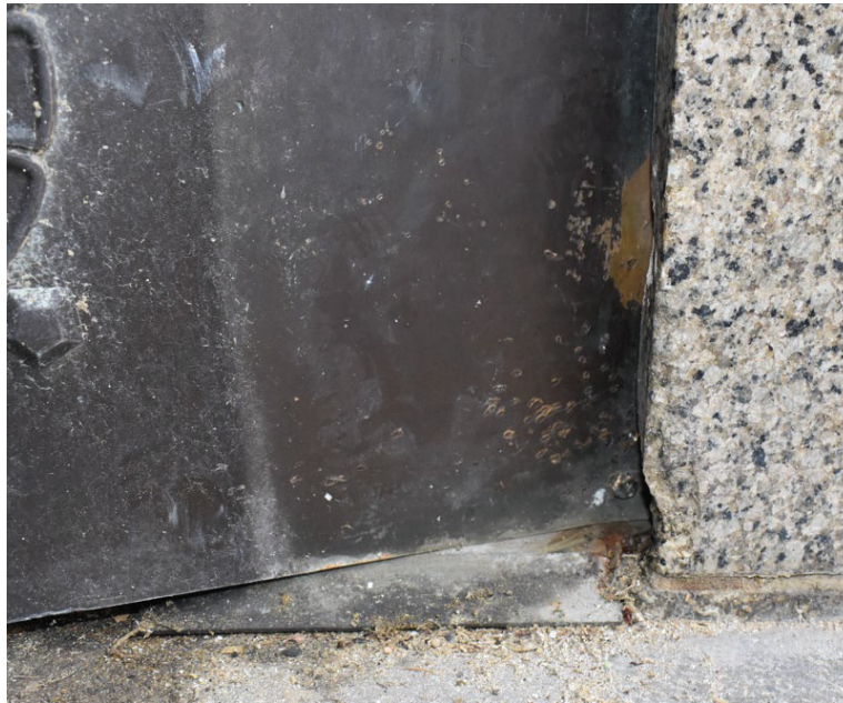
Detail image of deformation observed in the exterior side cladding. Image by TTG.
