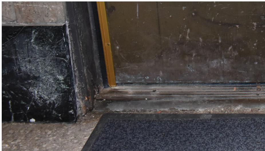
Detail image of lifting threshold observed during the assessment. Image by TTG.
