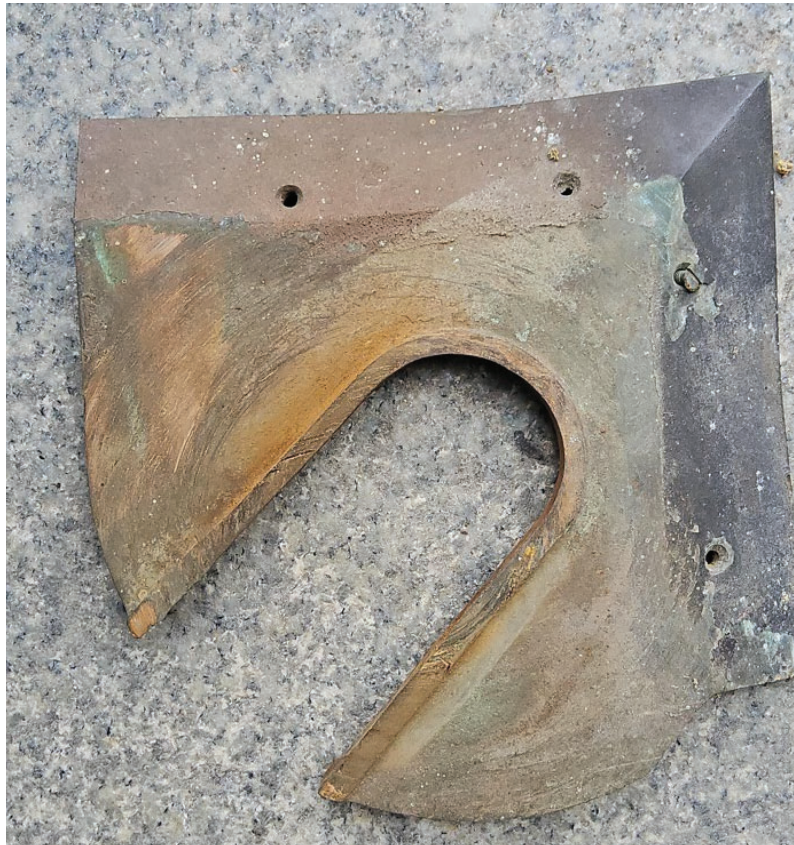
Detail image of an escutcheon plate removed during the assessment. Image by TTG.
