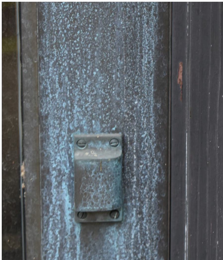
Detail image of green patina stains on the lower third of the interior door surface. Image by TTG.
