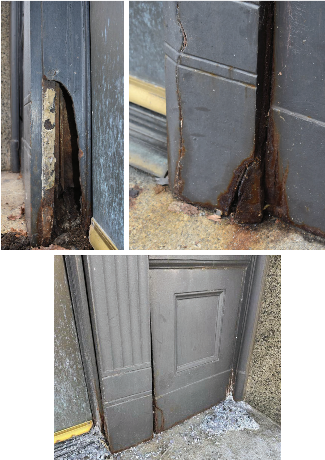
Detail images of deteriorated and corroded cast iron members. Images by TTG.
