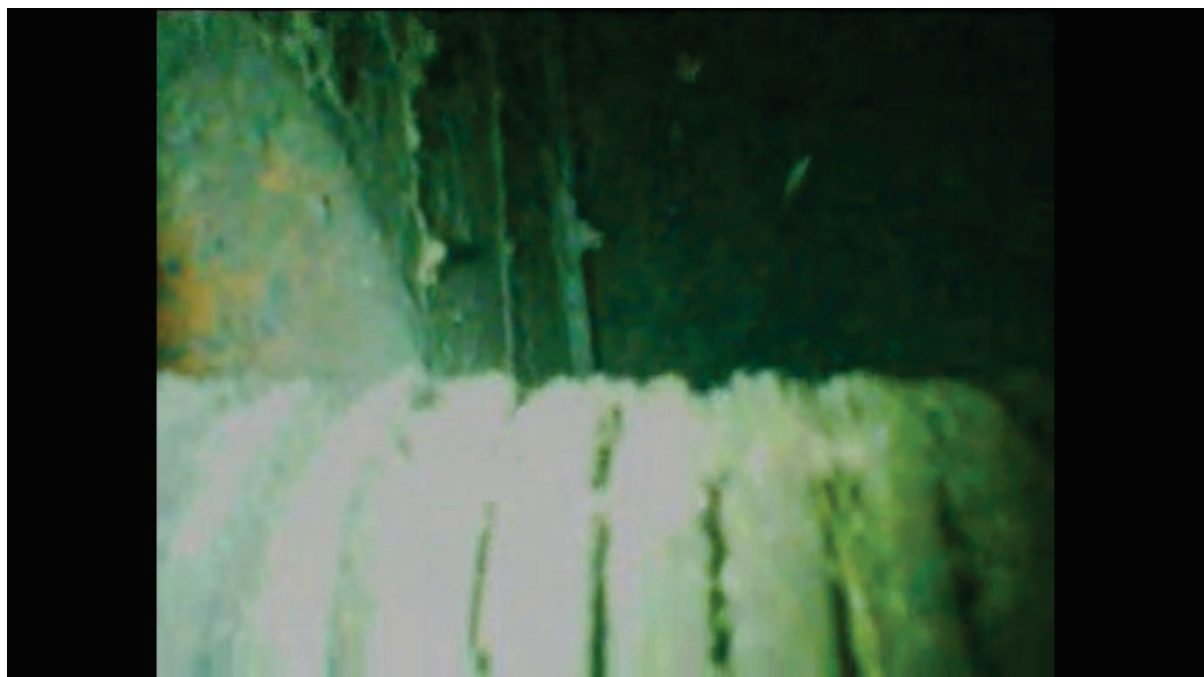
Borescope images of the internal fasteners that are backed out of the hinge pin. Images by TTG.
