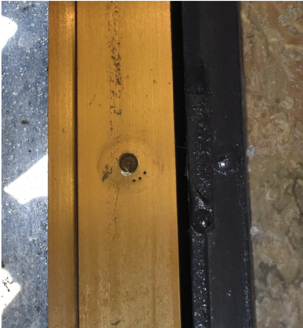
Detail image of the area where hardware is missing on the interior sidelight. Image by TTG.
