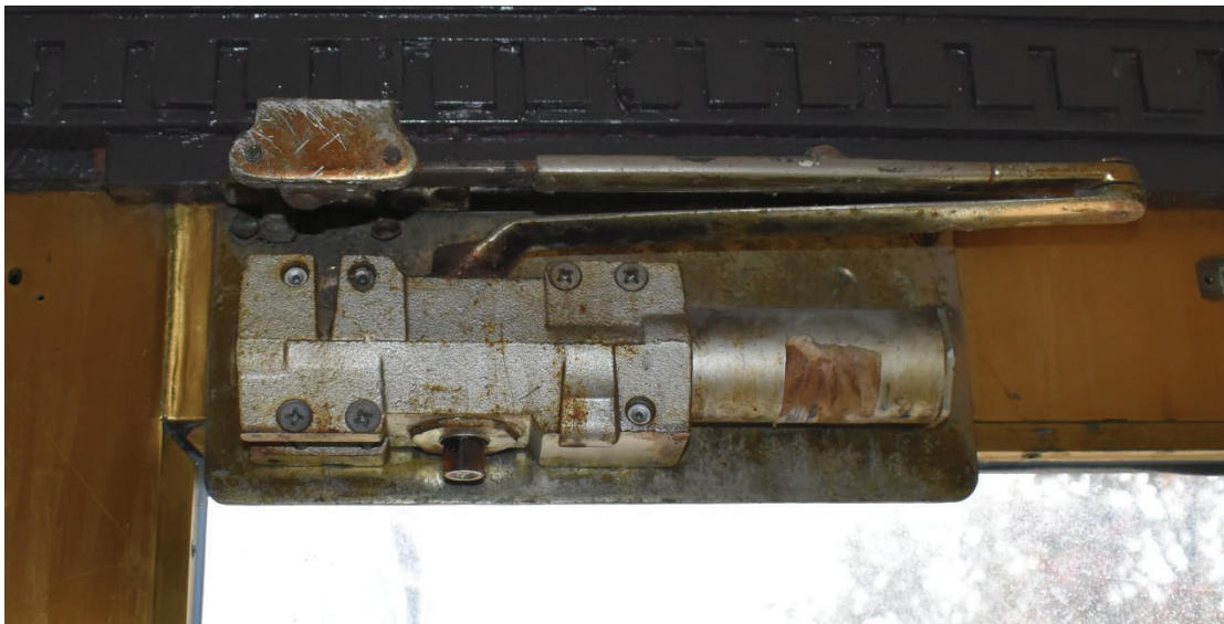
Detail image of semi-functional door closer. Image by TTG.
