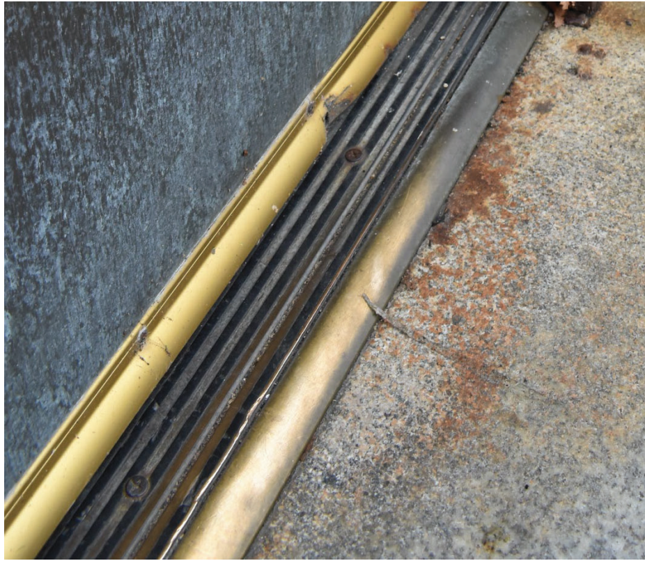
Detail image of deteriorated threshold. Image by TTG.
