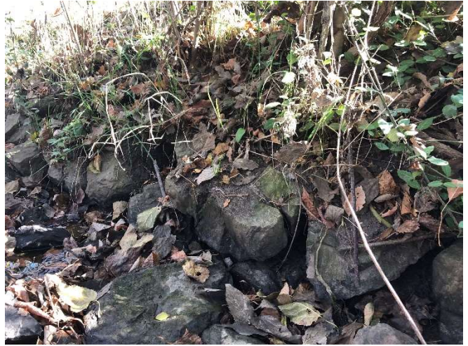
PRP 6 – Looking Upstream on UT1 Reach 2 showing armoring
