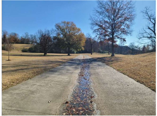
PRP 1 - Looking Downstream at oversized concrete channel on UT1 Reach 1
