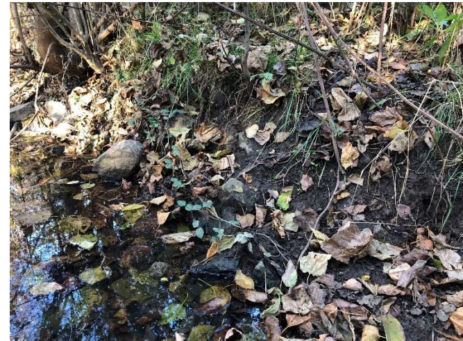
PRP 10- Looking eroding left bank on UT1 Reach 2
